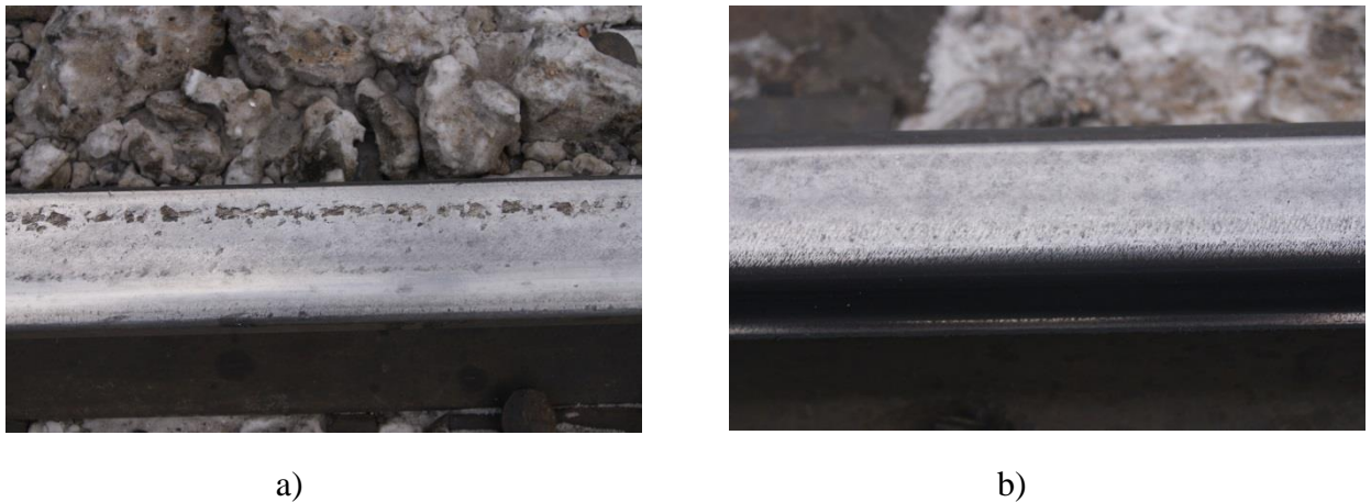
Figure 1.3. RCF damage of the rail 1 : a – subsurface; b – superficial
